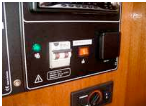
220-Volt Panel / FI Warmwasserboiler
